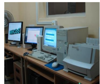
Mill Control Room
