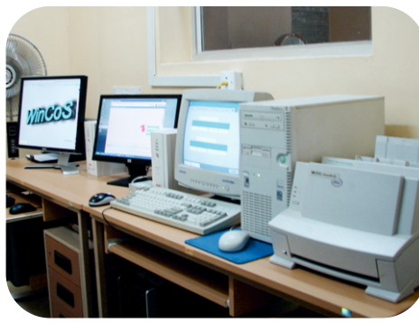
Mill Control Room
